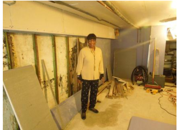
Deacon Carolyn Bolton during remodeling of the basement to become a pantry for the poor.
